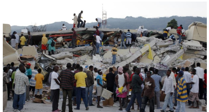
Earthquake in Haiti. [Online Image] Available http://s71165.gridserver.com , Feb. 2, 2010
